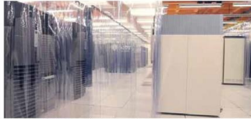
Energy optimisation - Vodaphone Datacentre France
